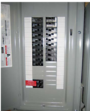
Figure 10: 70-Amp Double Pole Breaker. The electric service panel should have designated and labeled slots suitable for a 70-amp double pole breaker for use by the solar PV system.
