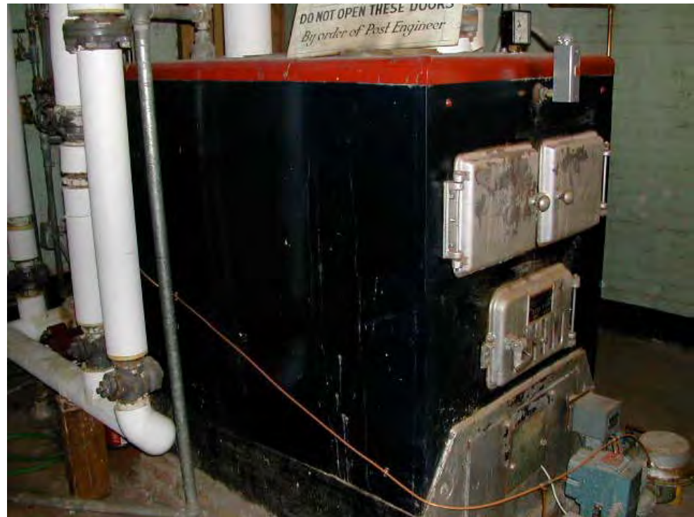
View of 1930s-era boiler
