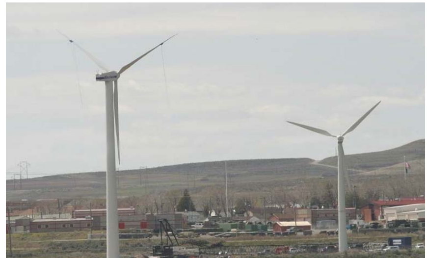
Figure 2 Newly installed Vestas V-47 660kW wind turbine at left and NEG Micon 225 kW wind turbine at right.
