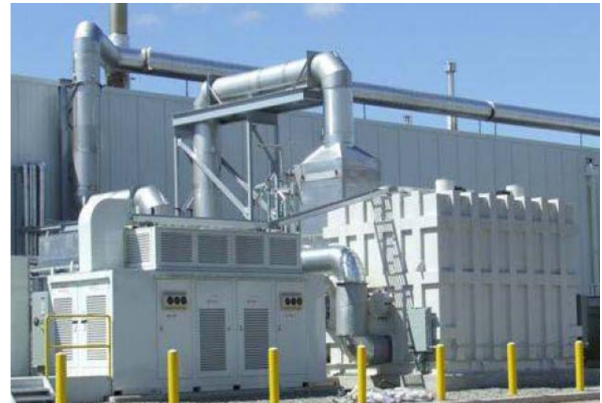
1500kW Carbonate FC Installation
