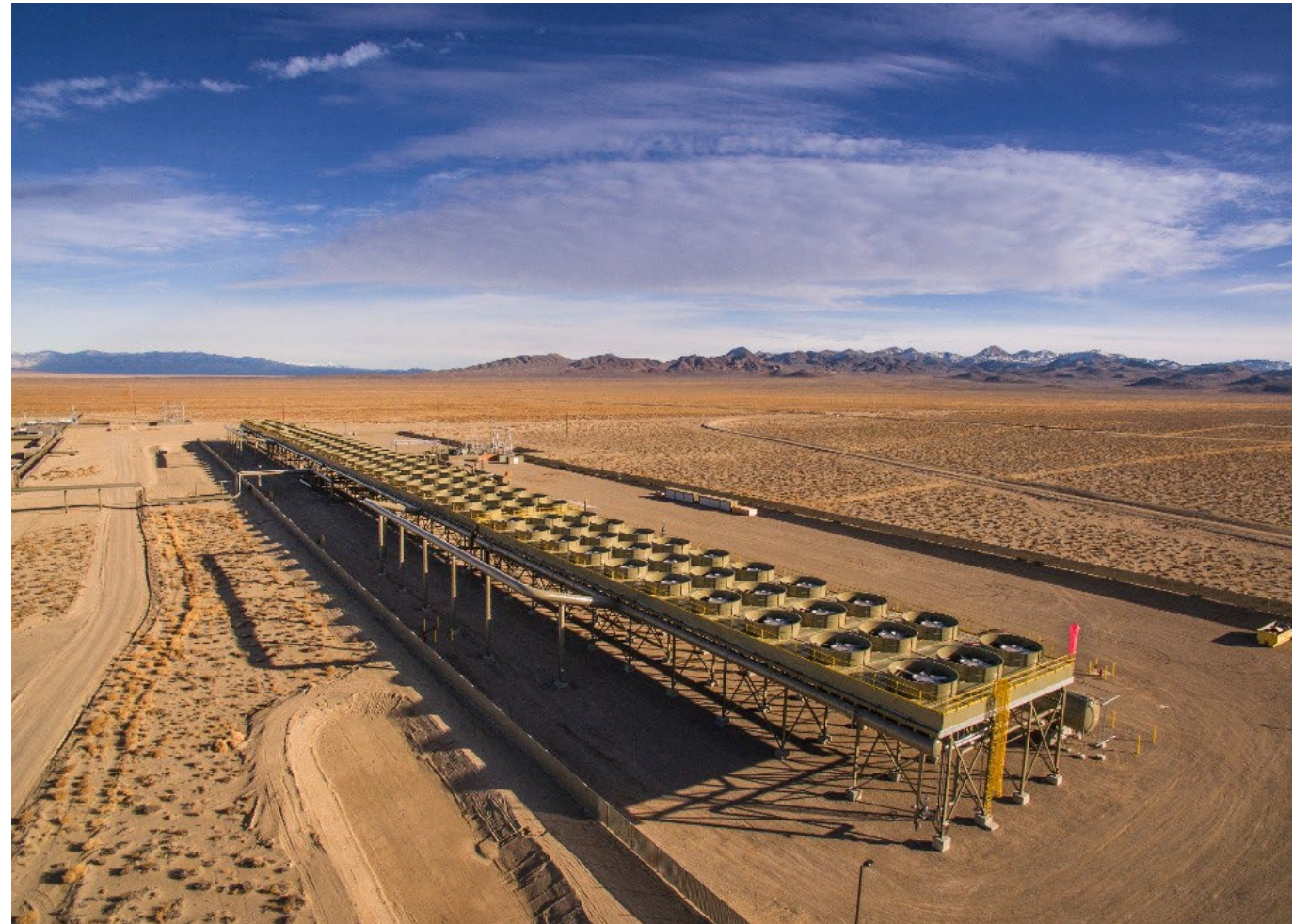
Ormat's 36 MW Don A. Campbell Geothermal Complex, Nevada, USA; a hidden system initially discovered during mineral exploration drilling
