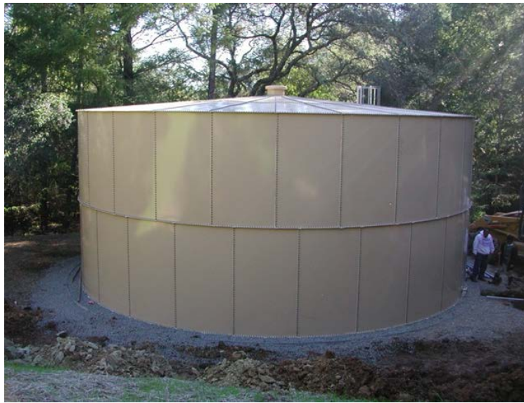
Figure 2-11. Steel water storage tank 99
