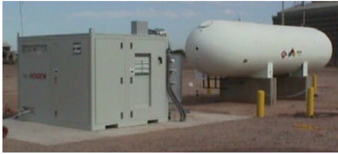
Figure 1 – Hydrogen Generator & Tank Installed in Arizona
