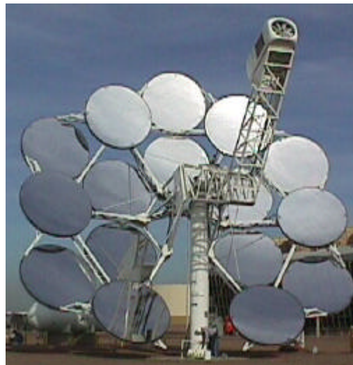
Figure 2 –SunDish System Installed in Arizona
