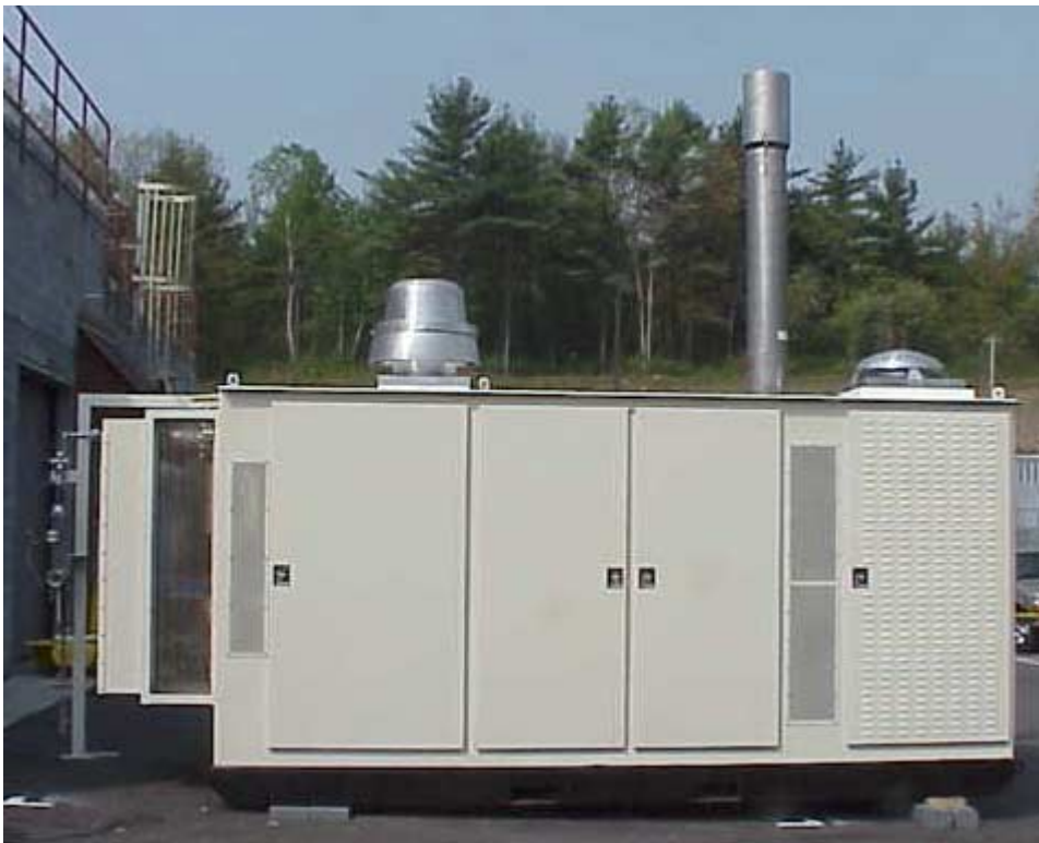
Figure 2 Plug Power Fuel Cell Power Plant
