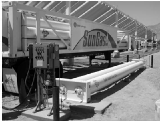
Figure 3. SunLine's FIBA tube trailer and ASME tanks for CH 2 storage
