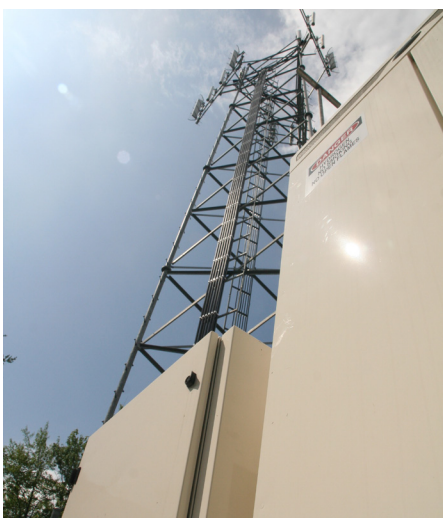
PlugPower fuel cells provide reliable backup power to cell phone towers.
