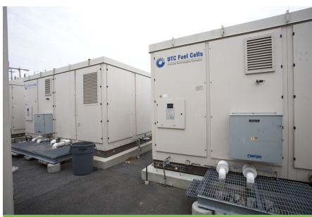
A fuel cell CHP system provides primary power, heating, and cooling for Verizon's Central Office.
