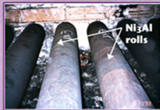
Nickel aluminide rolls show no sign of blistering in austenitizing furnace at 160" plate mill in Bethlehem Steel Burns Harbor Plant
