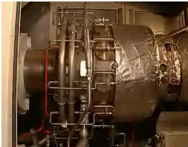
SC Johnson's Methane-fired Combustion turbine
