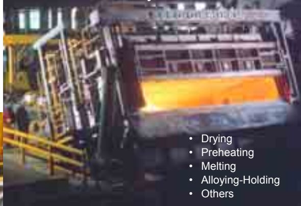
Gas Fired Reverberatory Aluminum Melter
