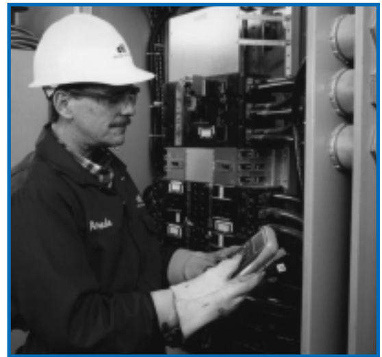
Motor load measurements quantify energy savings.
