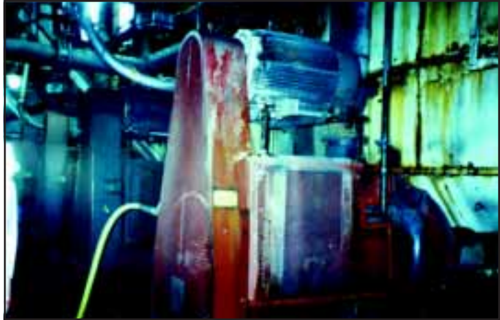
Coal Slurry Pumping System
