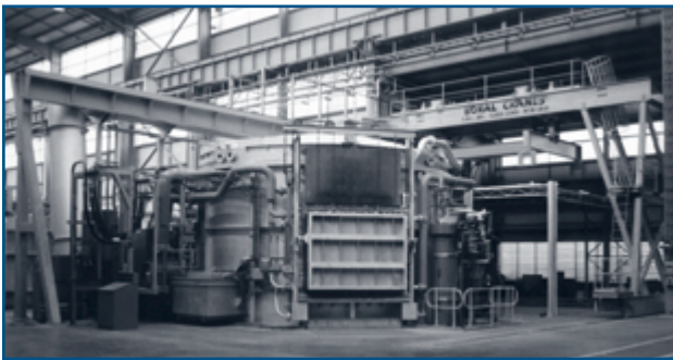
Tiling Top Aluminum Melting Furnace
