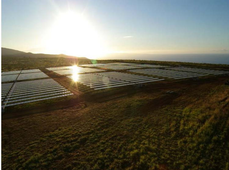
Figure 3: 1.43-megawatt (MW) PV system on Lana'i, Hawai'i
