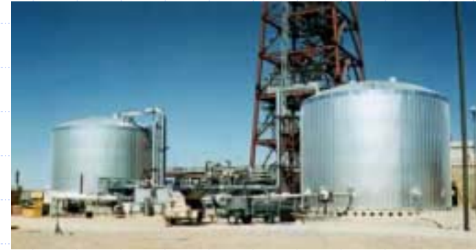
Solar Two Molten Salt Thermal Storage
