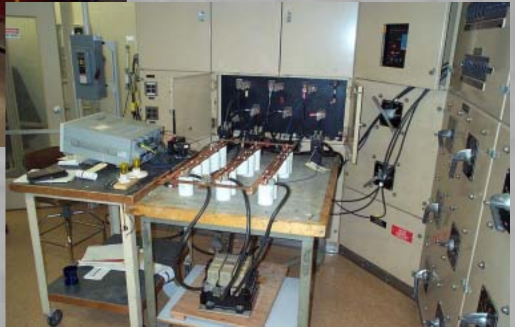
Capacitive Load Bank for Anti-Islanding Test
