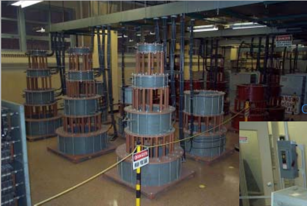
Inductive Load Bank for Anti-Islanding Test
