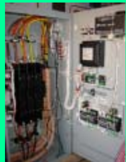
Switchgear, Relays, & Controls
