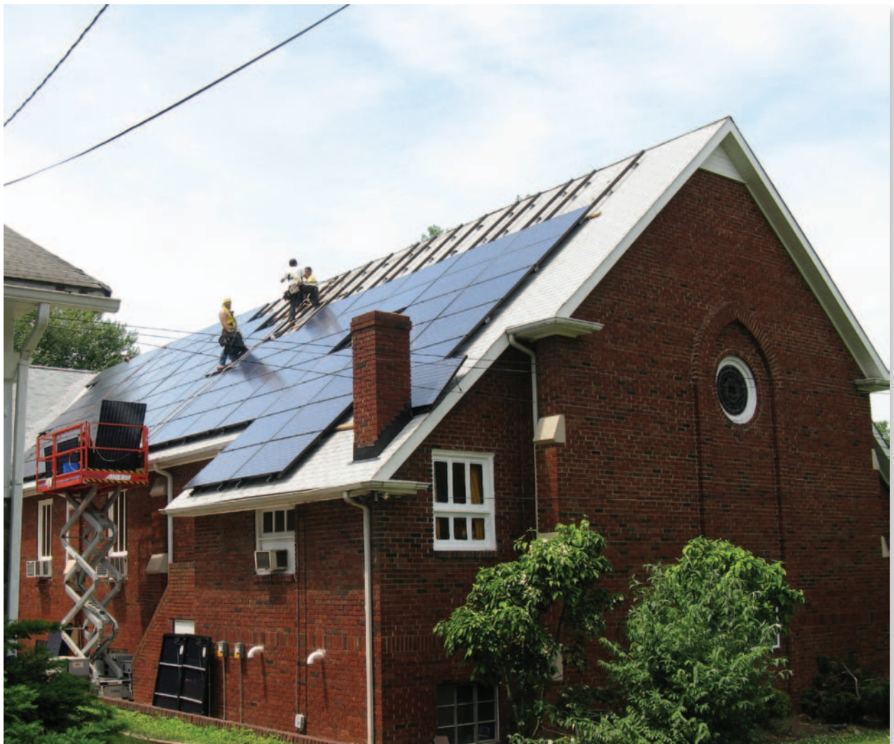
Panels on a Steep Roof, University Park, Maryland
