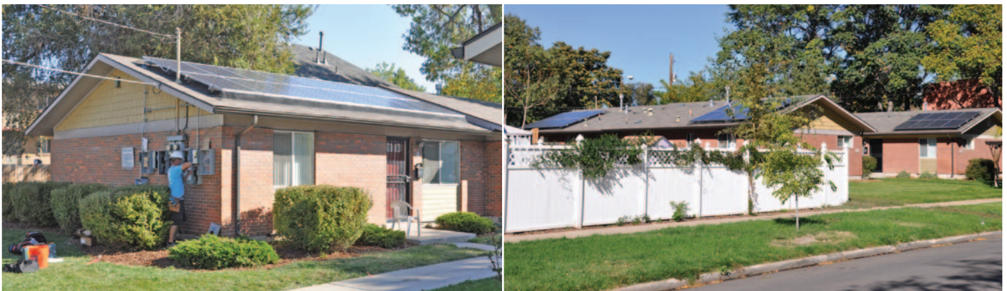
Figure 1. Single-story duplex PV systems. Photo from Northeast Denver Housing Center
