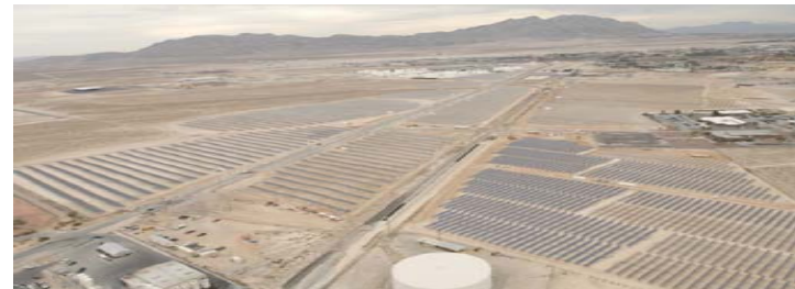
14MW PV Plant at Nellis AFB, NV (largest PV plant in the North America)
