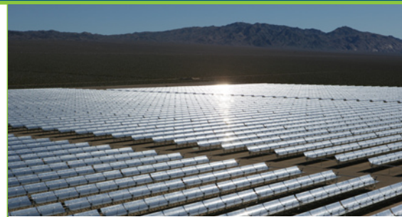
The 64-megawatt Nevada Solar One power plant went on-line in June 2007 (Photograph provided courtesy of Acciona).
