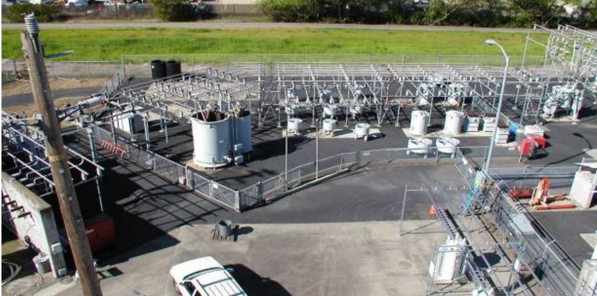
Figure 2-8. DUIT Test Facility, PG&E, San Ramon, California
