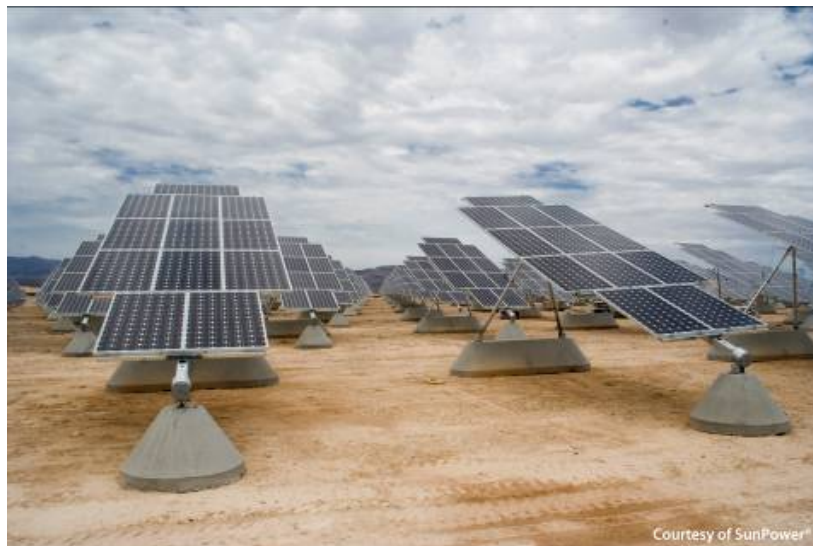
Figure 5-1. Nellis SunPower PV System
