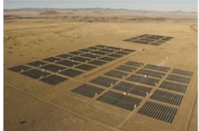
Fig. 1. Springerville PV Generating Plant
