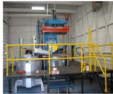
Low Pressure Casting Cell
