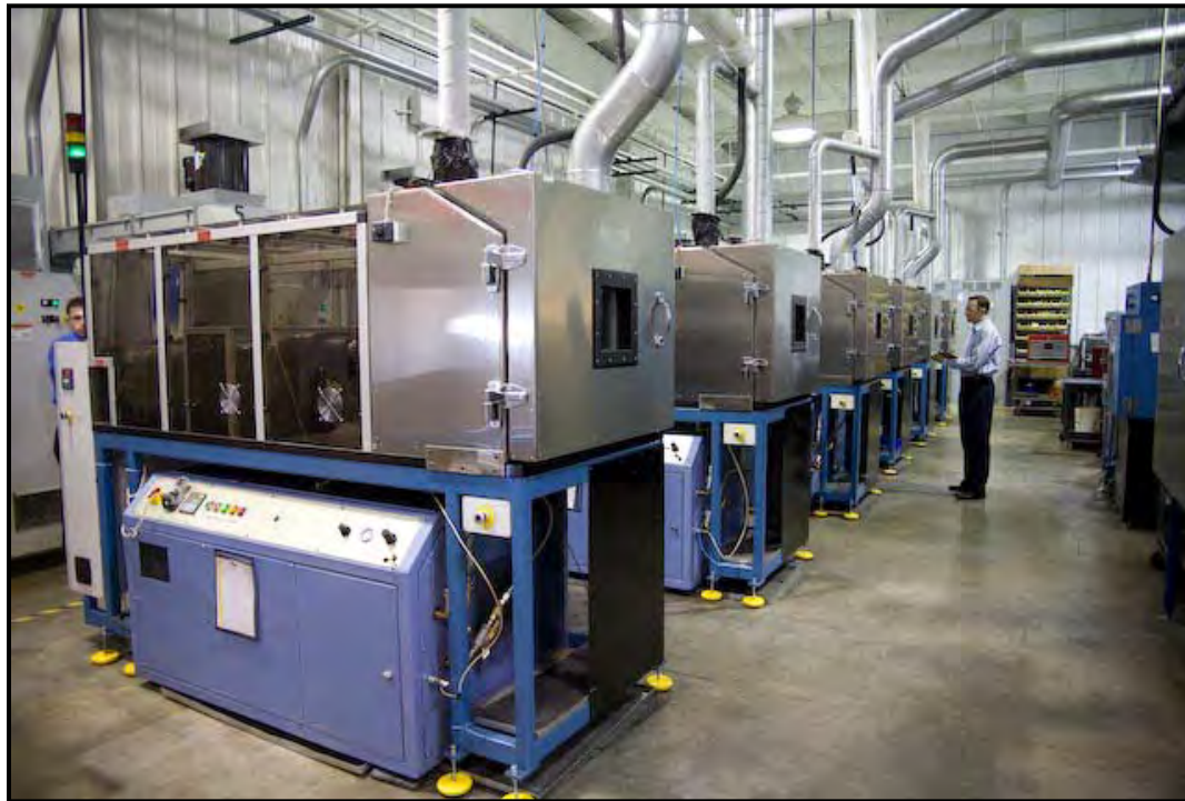
Motor Test Stands
