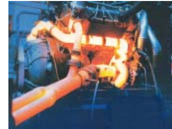
Exhaust System Waste Heat
