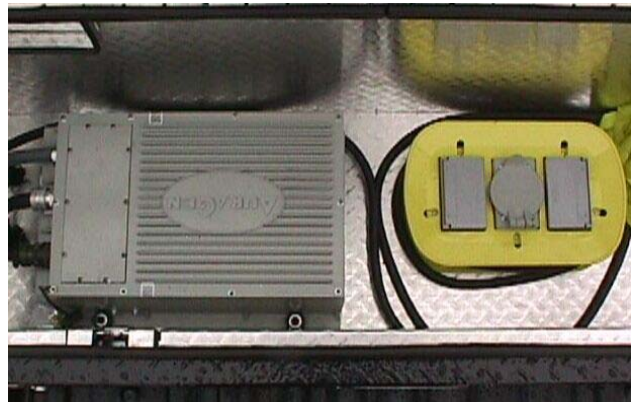
Figure 7. Onboard generator to supply power to the microwave system for the microwave-regenerated diesel particulate filter on the Ford 7.3-L test truck.
