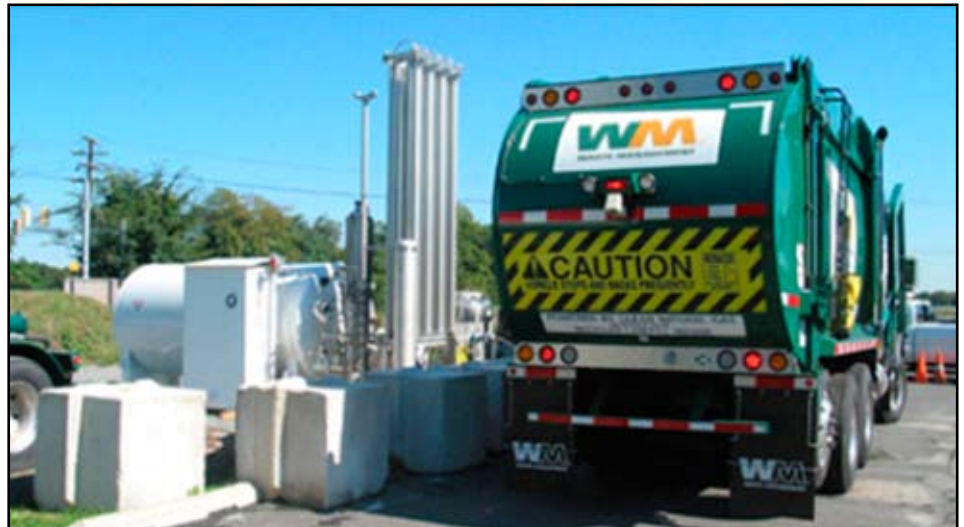
LNG storage tank and fueling station (Photo courtesy of Acirion)
