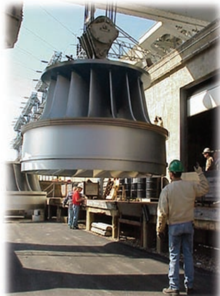
Workers lower a new hydropower turbine to be installed as part of the Osage Project at the Bagnell Dam on Missouri's Lake of the Ozarks.
